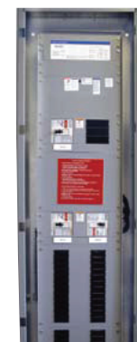
Wall-mount maintenance bypass panel
